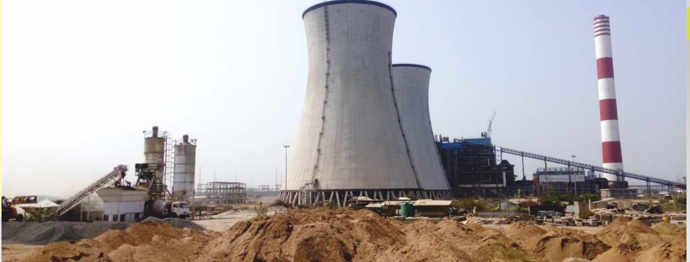
M1 Batching Plant at Bhavnagar Energy Company Ltd Thermal Power project by Shapoorji Pallonji
