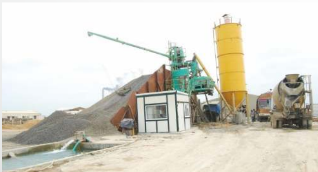
TATA Power Gammon CP 18 with star batcher at Mundra Power project
