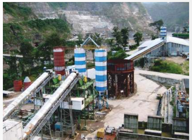
H6N batching plant at Subansri where 10 0 centigrade concrete was supplied through a belt conveyor
