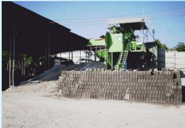
CP 30 Batching plant
